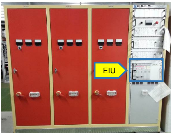
Fig.2 SR PS power supplies (3 units in a single cabinet)
